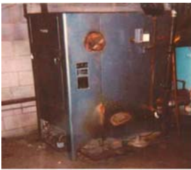
Boiler Explosion-Day Care Facility Minnesota Department of Labor & Industry Investigation
