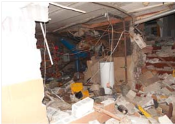
This picture shows what is left of the wall that separated the boiler room from the north/south hallway.
